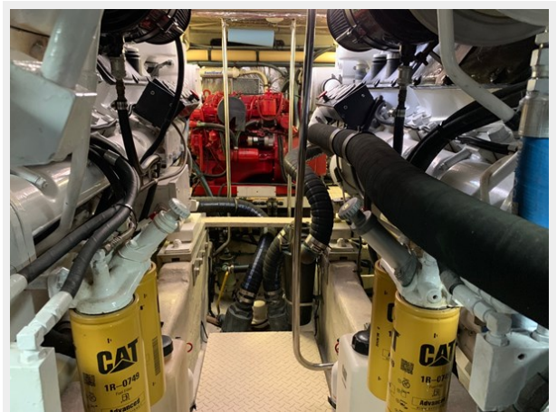
1995 SEA RAY 63 ENGINE ROOM
