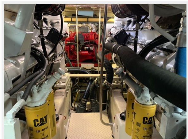
1995 SEA RAY 63 ENGINE ROOM
