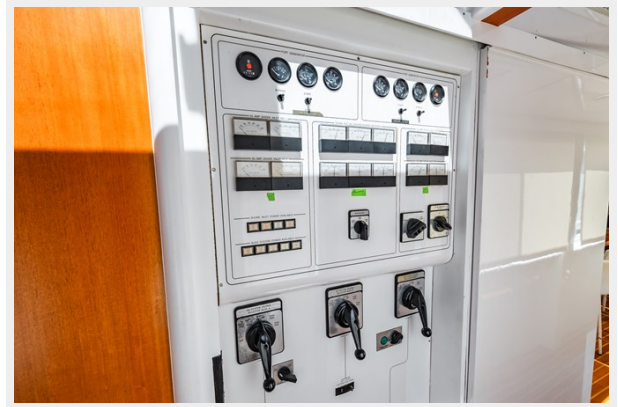
Companionway Switch Panel
