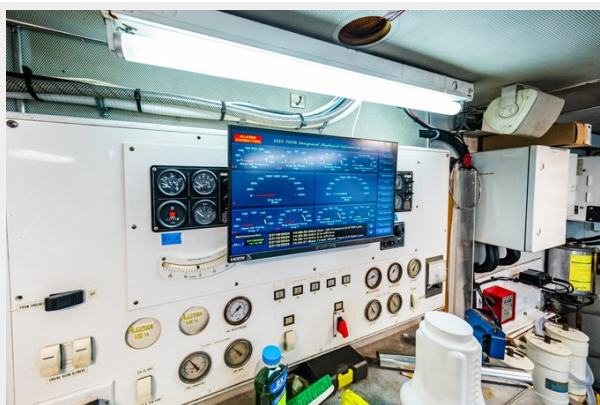
Engine Room Center
