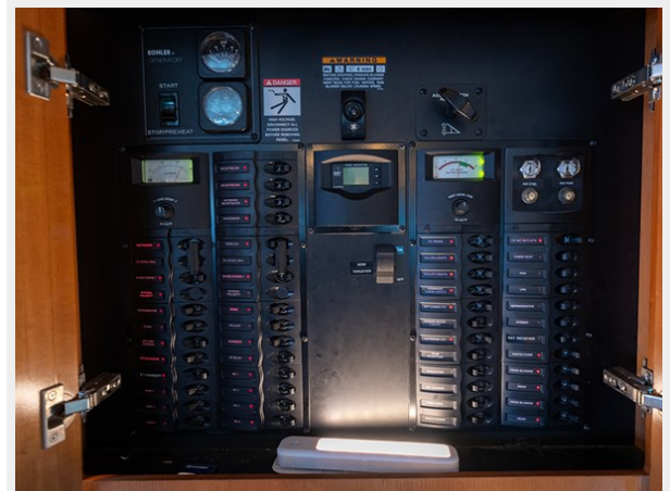
Main distribution panel
