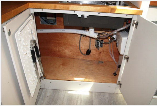
Storage under Galley Sink
