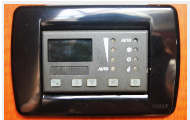
AC/Heat Control in Cabin
