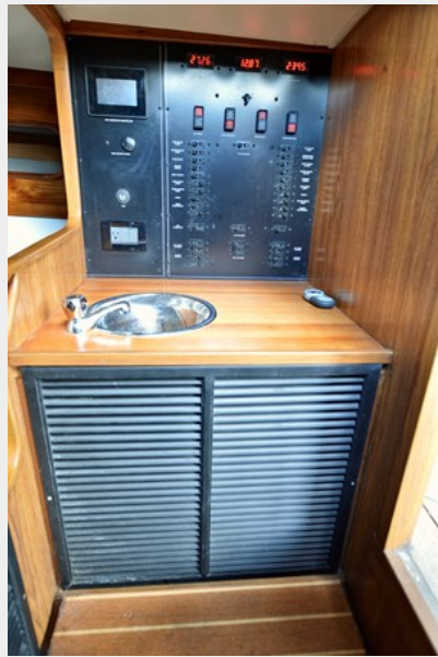
29 STRIKE 2023 MAIN BREAKER PANEL
