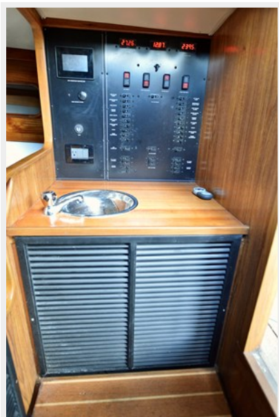
29 STRIKE 2023 MAIN BREAKER PANEL
