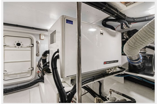
Generator port side aft
