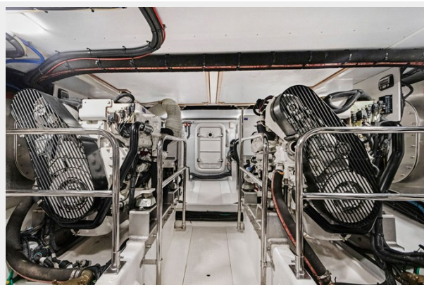
Engine room looking aft
