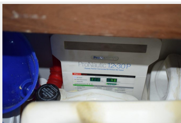
Battery Charger Beneath Cabin Step
