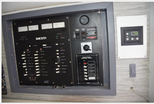
Main Electrical Panel and A/C Control
