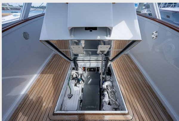
Engine Room Access
