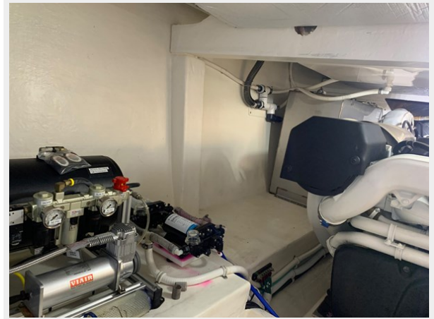
Engine Room Starboard
