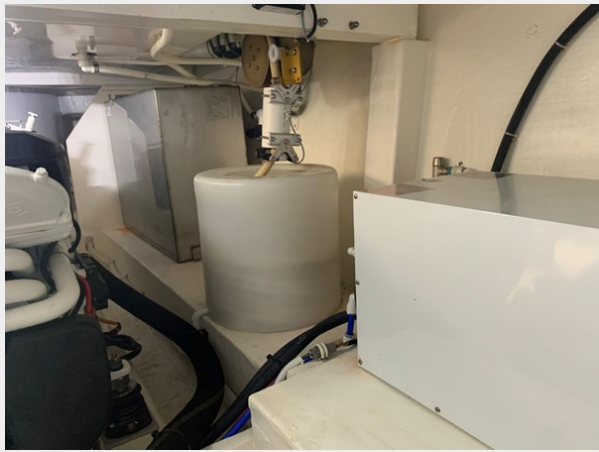
Engine Room Port
