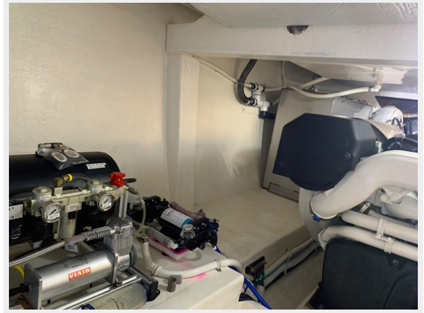
Engine Room Starboard
