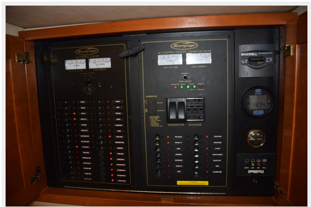
Primary Electrical Panel
