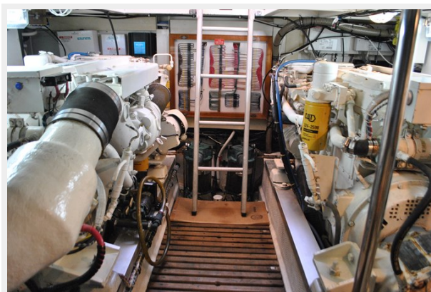
Engine Room Forward View
