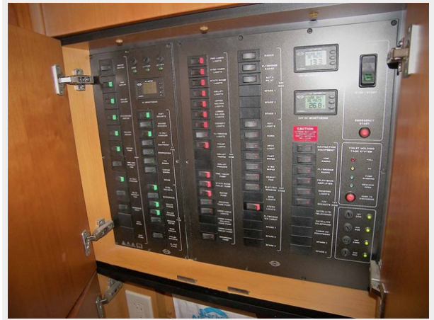
Main Electrical Panel
