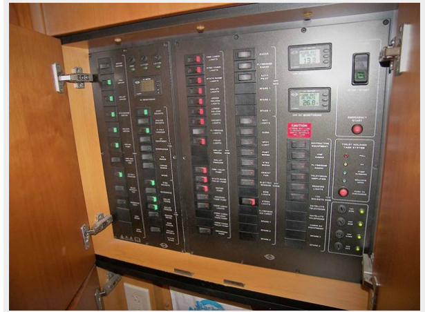
Main Electrical Panel
