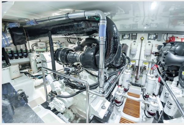
Engine Room Facing Portside
