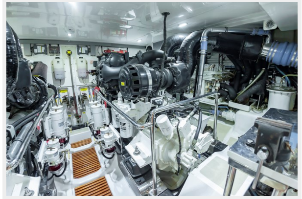
Engine Room Facing Starboard
