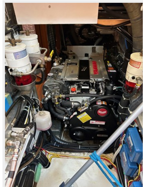
Engine Room Forward
