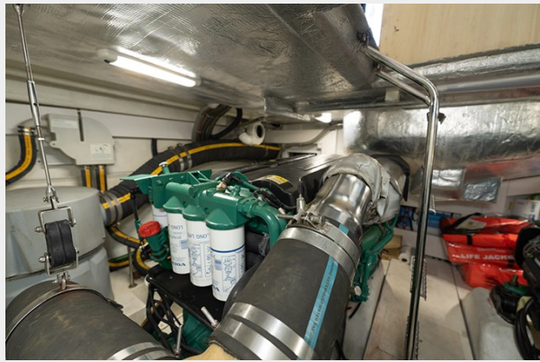
Engine room view 2
