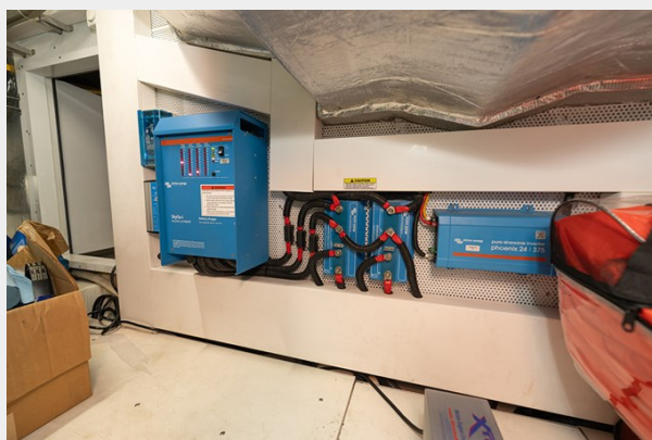
Engine room view 4
