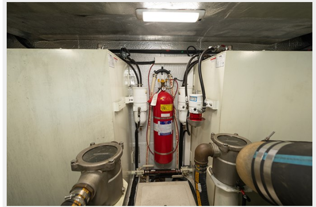
Engine room view 3
