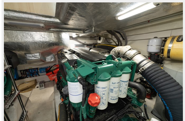
Engine room view 1
