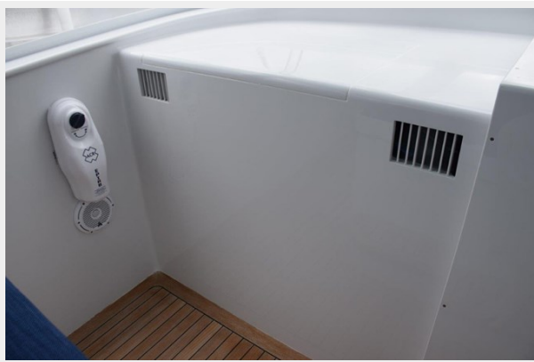
Helm air conditioning and EPIRB
