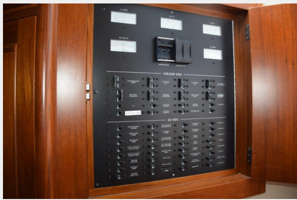
Main electrical panel
