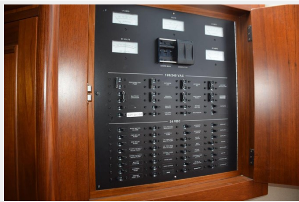
Main electrical panel
