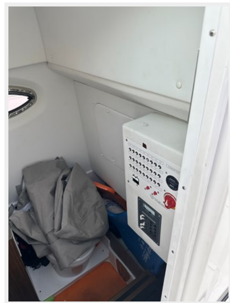
16. 302 head shot battery switches
