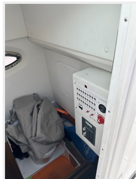
16. 302 head shot battery switches
