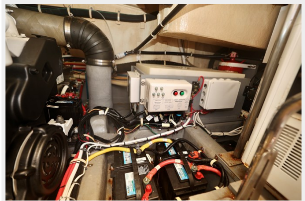
43 CARVER 2015 ENGINE ROOM 2
