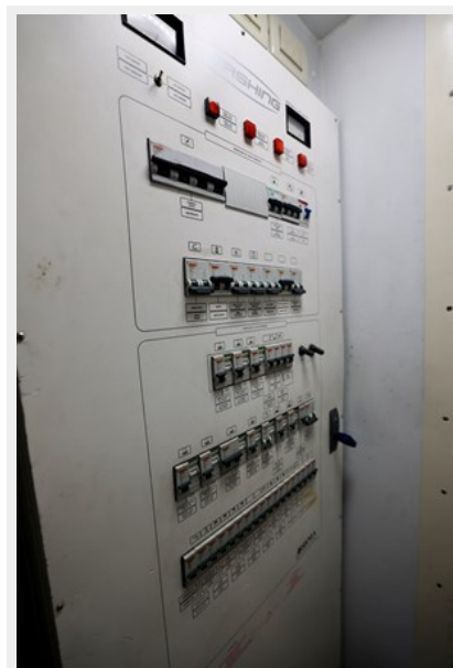
72 PERSHING 2009 MAIN ELECTRICAL PANEL
