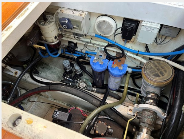
Pump and pit area
