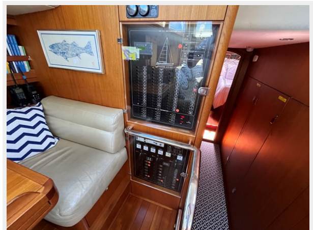
AC and DC distribution panel
