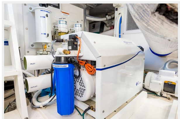
Maritimo M51 Engine room
