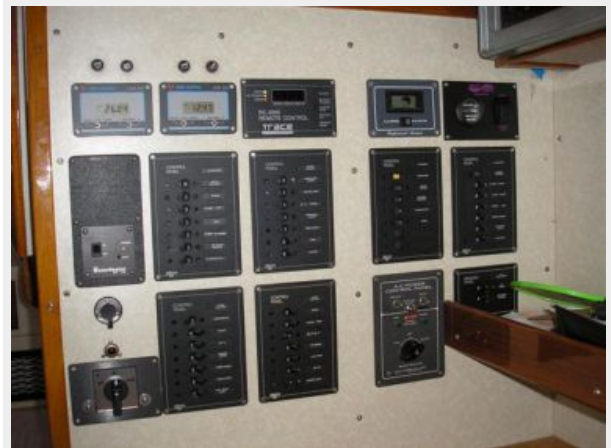
Electrical Panel at Navigation Station
