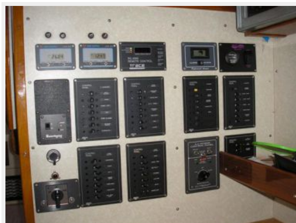
Electrical Panel at Navigation Station
