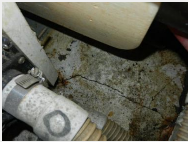
crack in concrete
