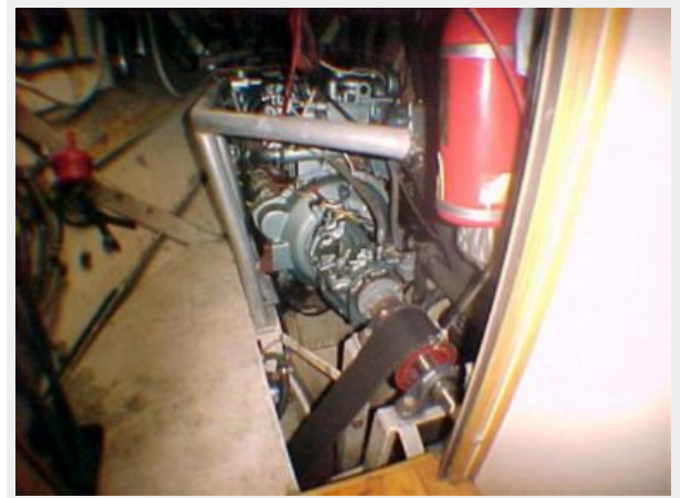
Engine room entry
