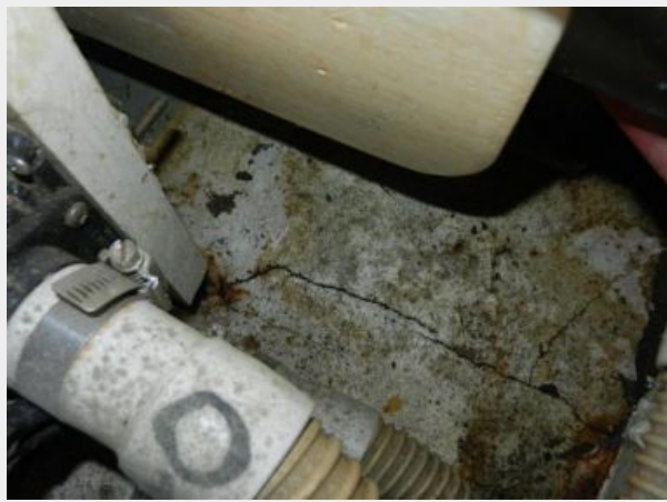
crack in concrete
