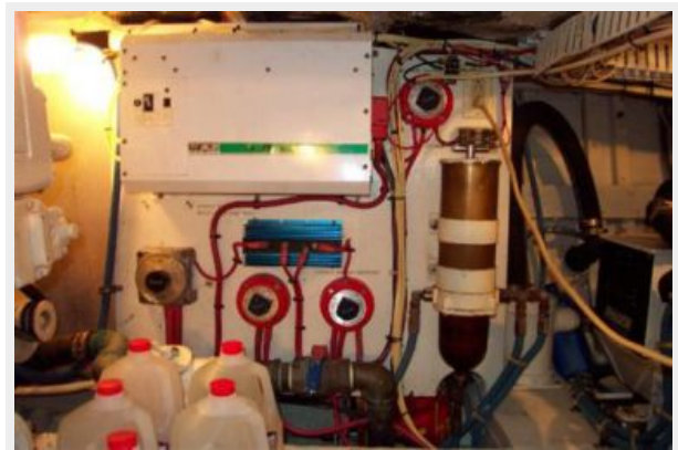
Port Engine Room
