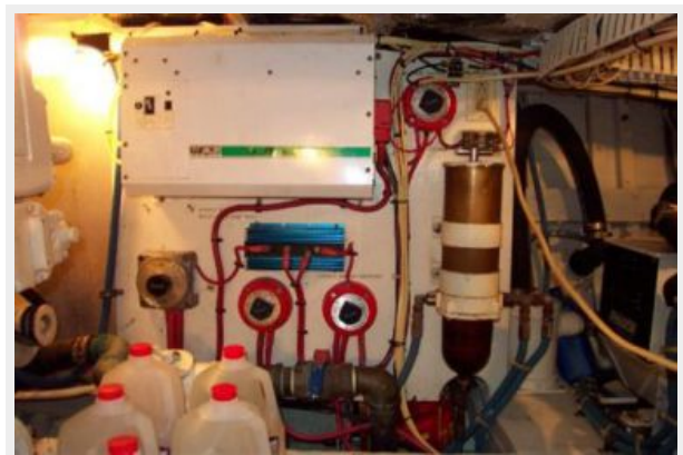
Port Engine Room
