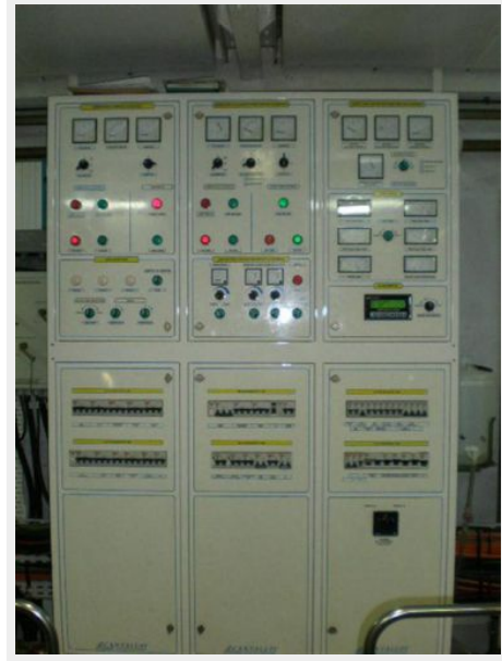
Machinery control panel
