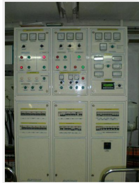
Machinery control panel
