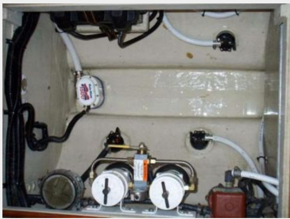
Clean Port Bilge
