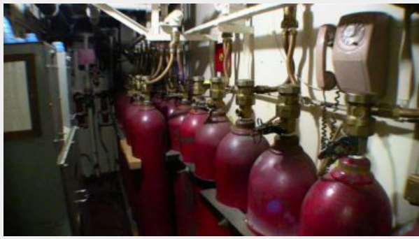
C02 fire control
