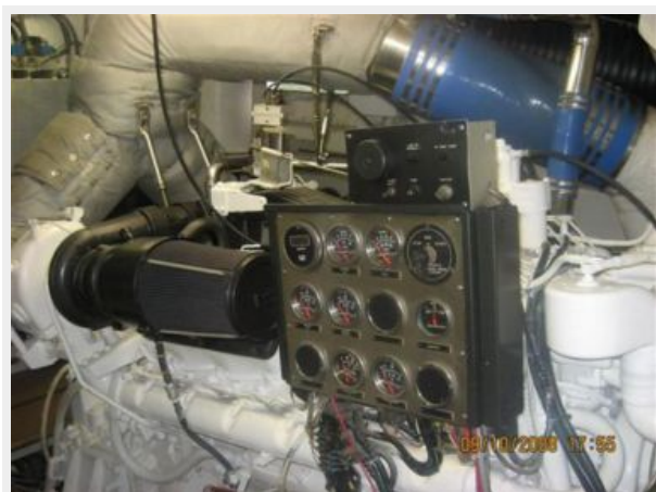
Starboard Main Engine
