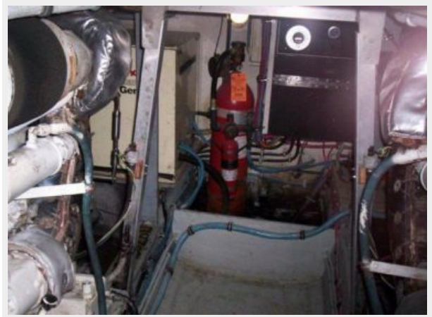
Engine & Mechanical Equipment
