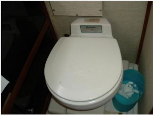
Fresh water flush toilet
