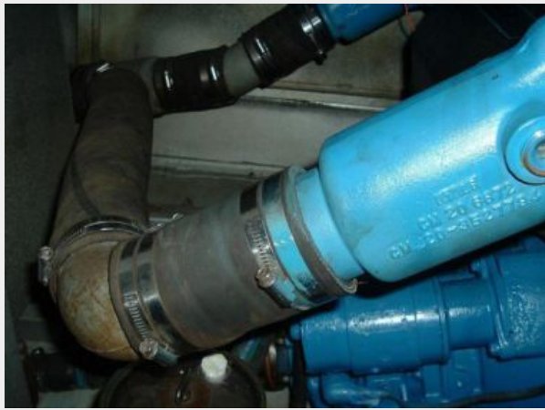
Port Motor Exhaust Tubes
