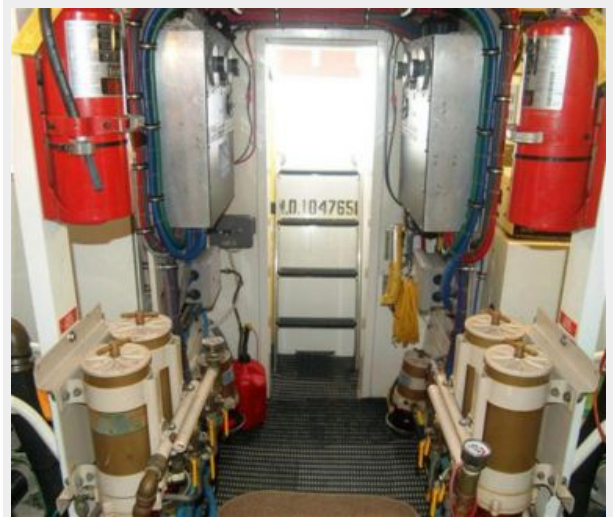
Engine room looking aft
