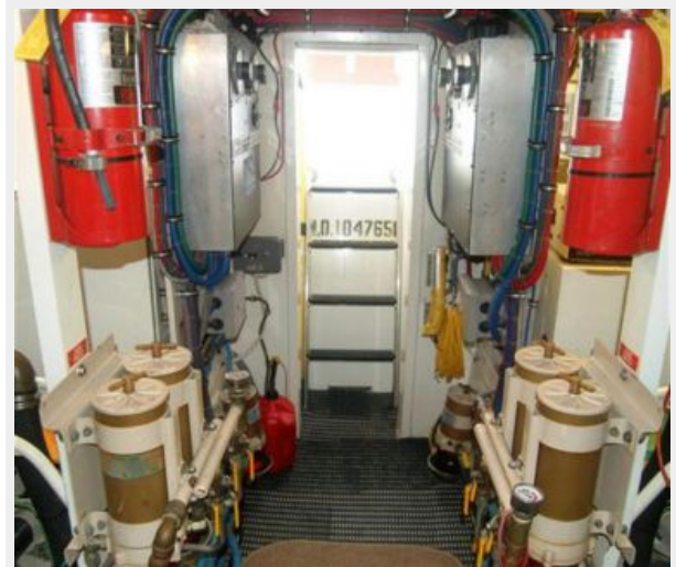
Engine room looking aft
