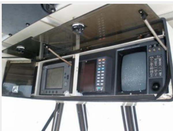
Bridge Electronics Box
