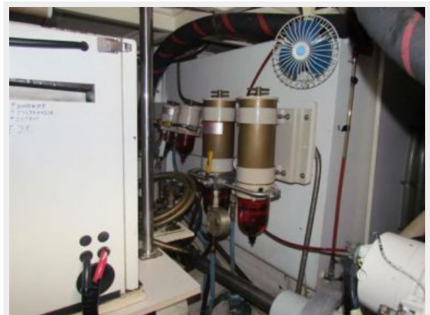
Starboard Fuel Tank
