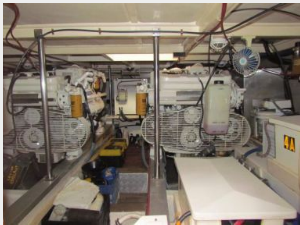
Engine Room Aft
