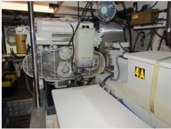
Engine Room Aft
