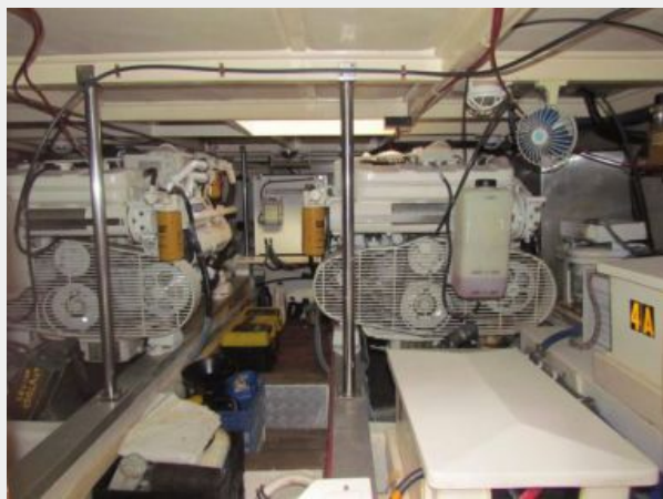
Engine Room Aft
