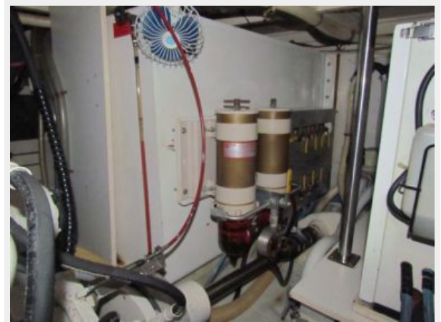
Port Fuel Tank
