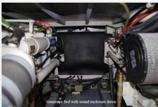
Engine Room From Cockpit Entrance
